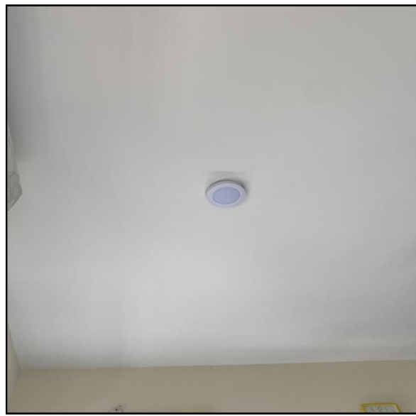
Efficient light (LED Downlighter)
