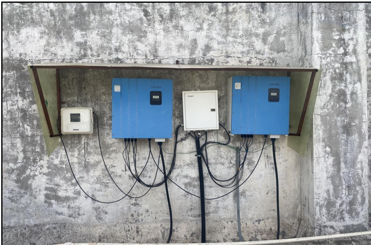
Figure 2.4:- Solar plant 480 KWp and inverter system
