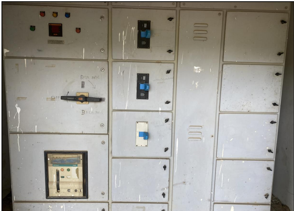
Figure 2.3 Capacitor bank on main panel
